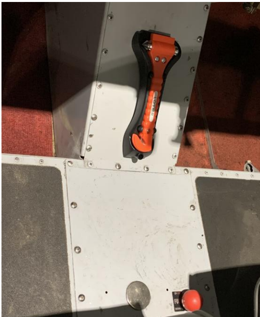
FIGURE 7-11 EXAMPLE EGRESS HAMMER INSTALLTIONS
